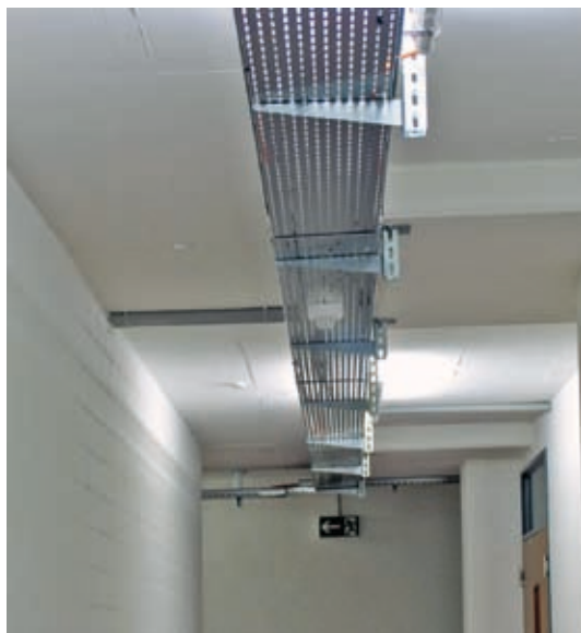
Corridor with cable route
